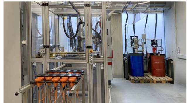
The refill unit of the new encapsulation station is located directly next to the dosing/mixing system, and robotic cell and ensures reliable replenishment of synthetic resin and hardener .
