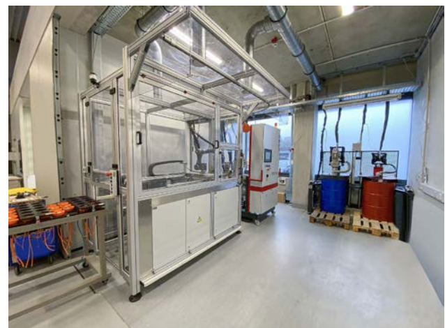
Implemented TARTLER GROUP companies: Fully automatic system solution consisting of dosing and mixing unit, encapsulation station and refilling unit.
